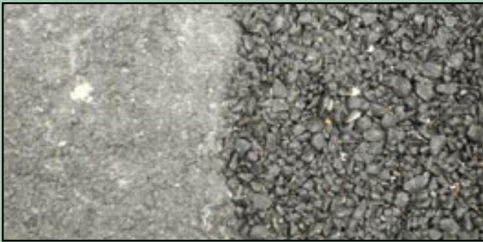
The comparison of traditional asphalt (left) and porous asphalt (right). Porous asphalt lacks the fine particles of stone and binder course that makes it impervious. Porous asphalt works very well; however, it is important not to use sand for de-icing as that will clog up the pores. It is recommended that once a year the surface be vacuumed to remove debris that has fallen on the site.
